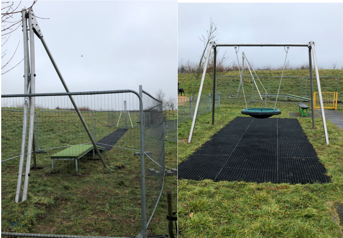
Photo of new zip wire and swing under construction at Bersted Park
