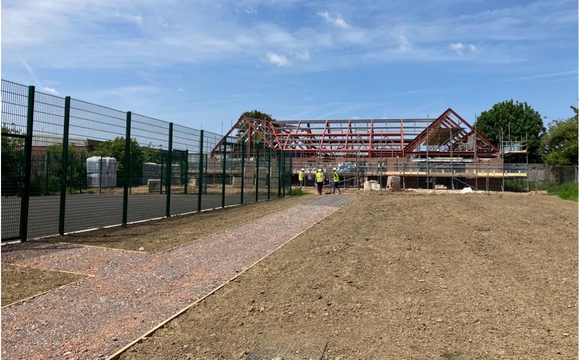
Photo of the new Keystone Centre and MUGA in Eldon Way Littlehampton under construction
